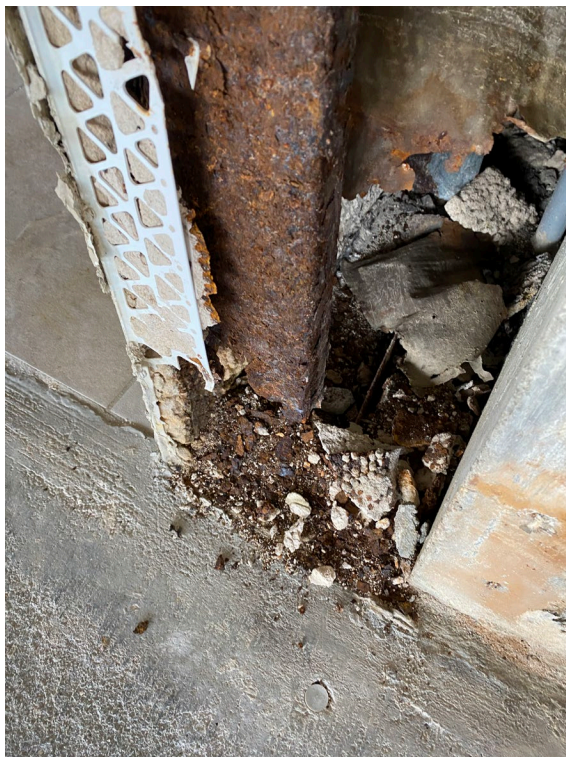
Picture 5: Corroded wall stud, East side of elevator lobby
