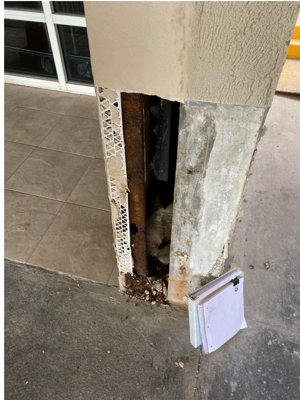
Picture 4: Corroded wall stud, East side of elevator lobby
